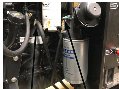
Fuel Return Line Connection
